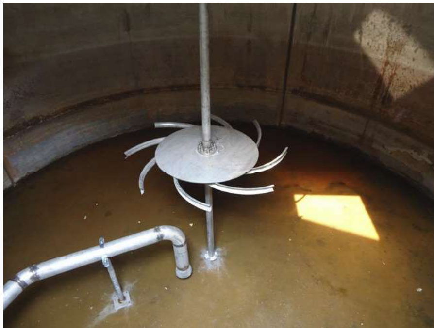
A high performance centrifugal dispersing impeller used for sludge mixing at the Banff WWTP.
